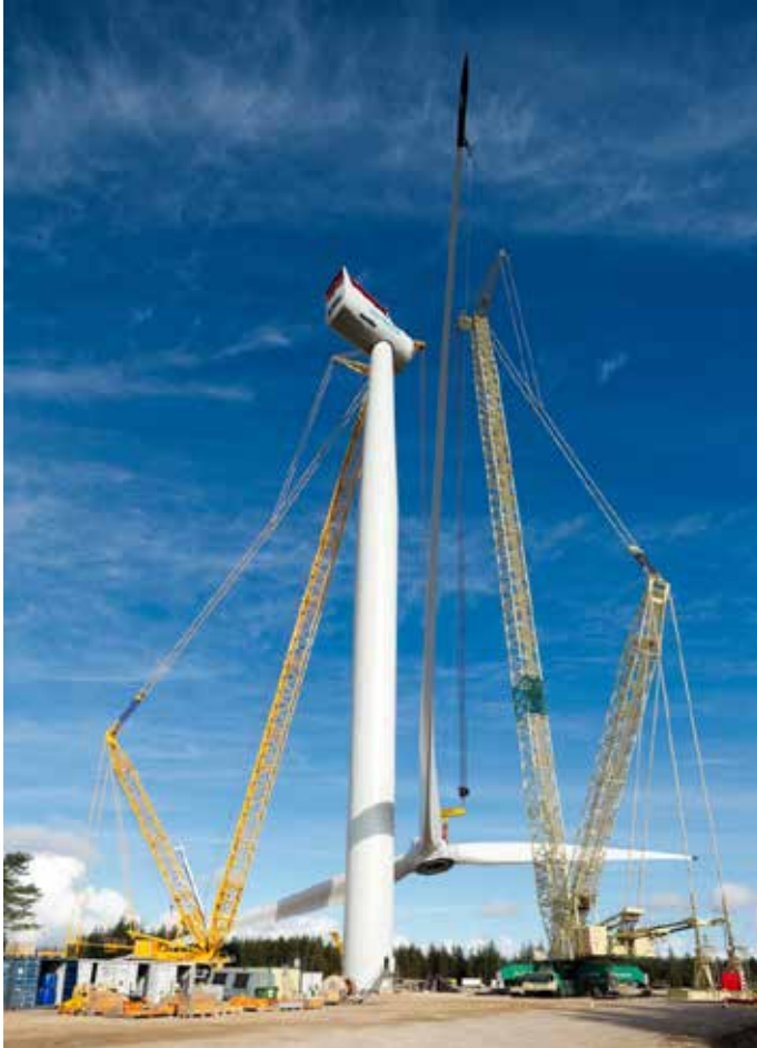
Source: Siemens Press Picture
