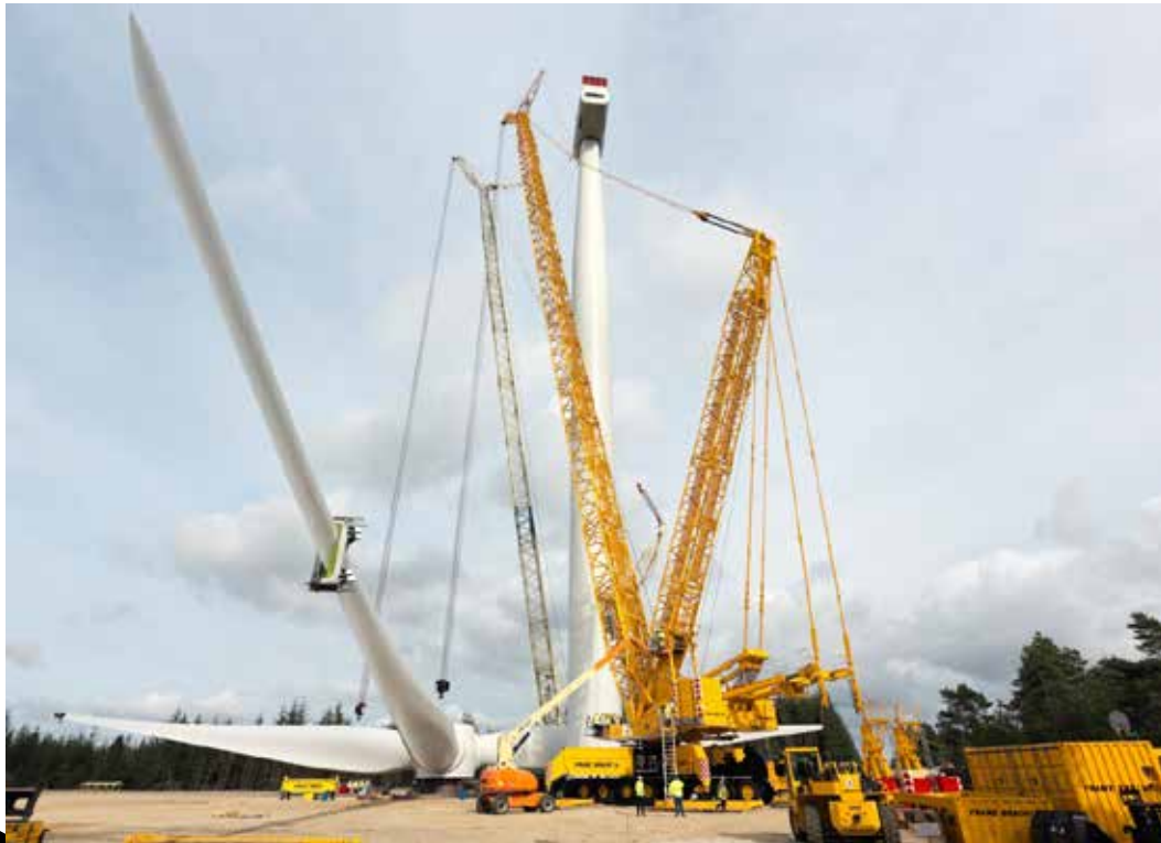
Source: Siemens Press Picture
