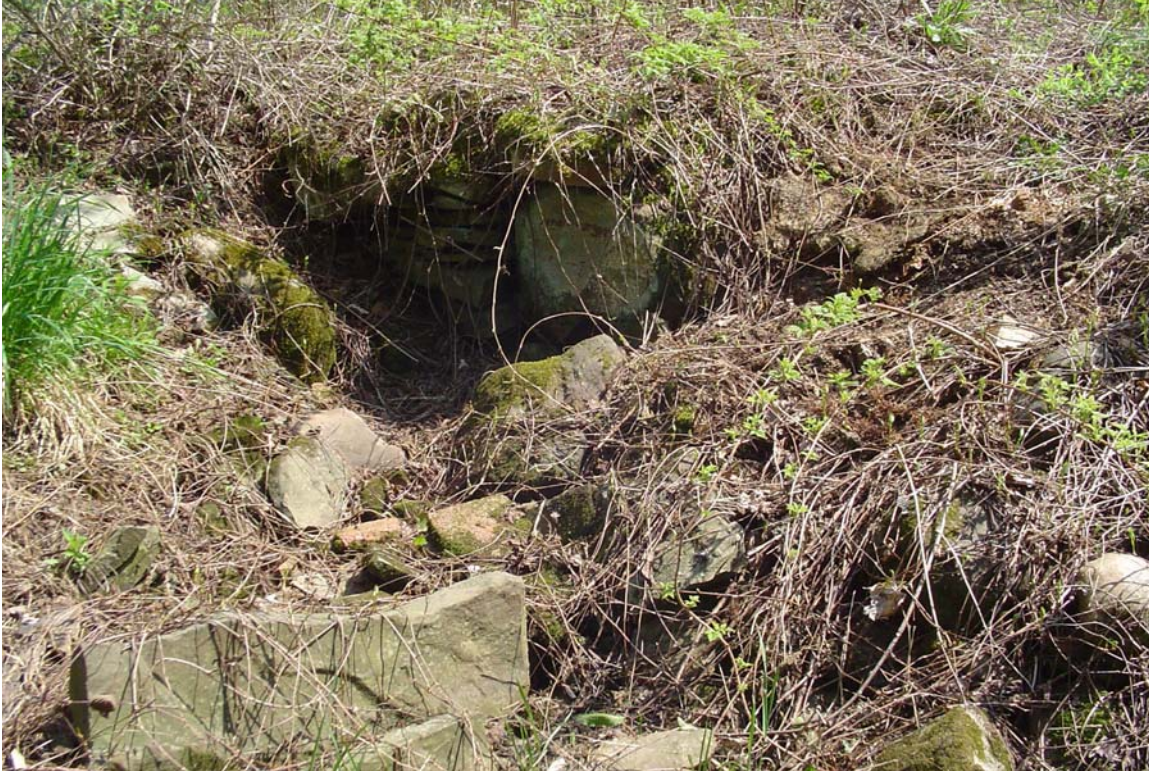
Photograph 15. Damaged foundation at Linear 13, facing northwest.
