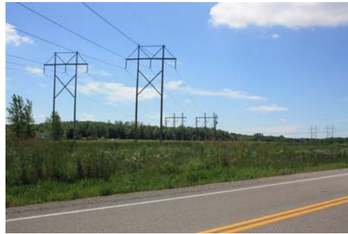
Existing Transmission Line
