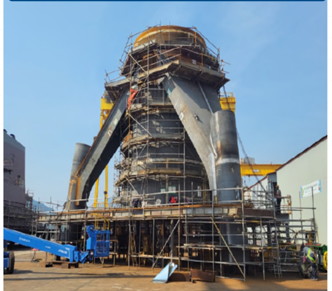
Transition piece of jackets are being completed and ready for final paint coat
